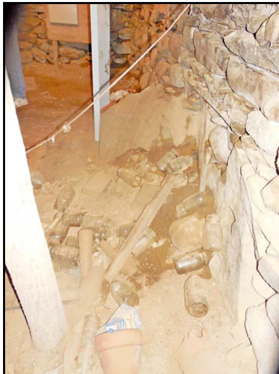
Photo P04 – Stone foundation wall with soil wash out accumulation.
