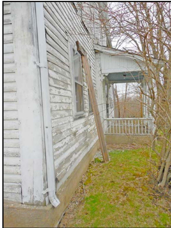
Photo P12 – Front wall at west side with modern concrete encapsulation base trapping moisture.
