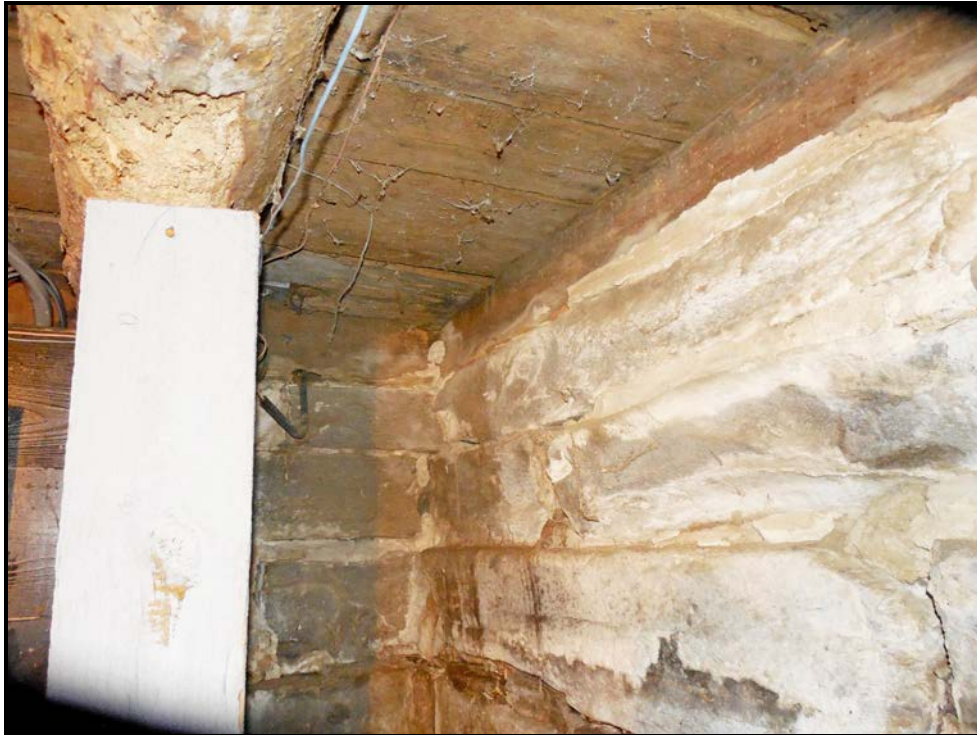
Photo P01 – Timber sill with mortar seal trapping moisture in wood.
