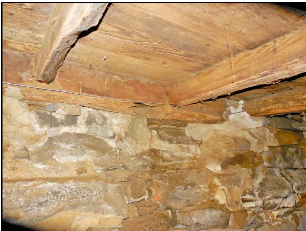
Photo P02 – Front timber sill with dry rot and powder post beetle damage.
