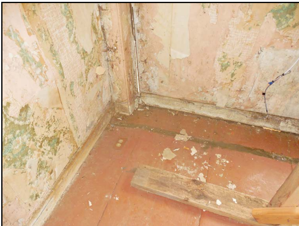
Photo P06 – Close up of damage at front parlor southeast corner. Note lateral movement at floor and light entry at post.
