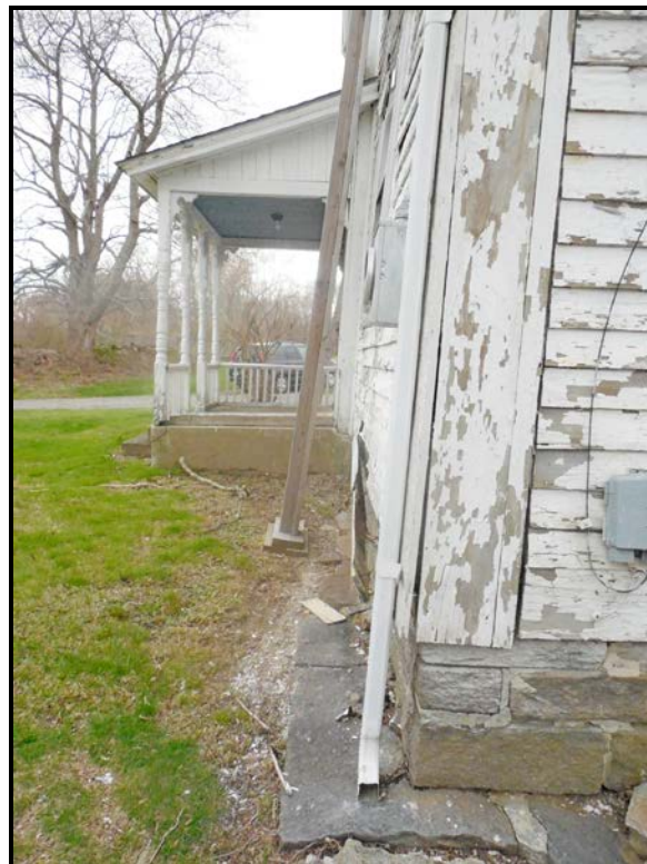
Photo P10 – Front sill/post damage and outward movement of wall base at southeast corner.
