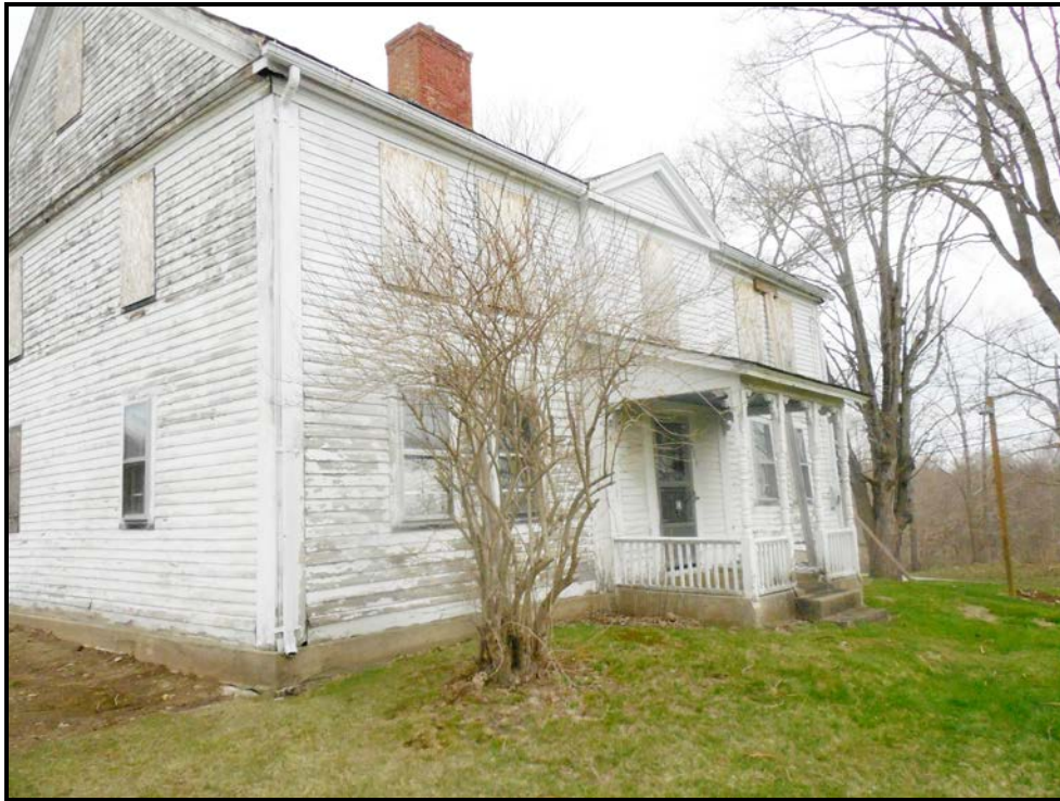
Photo P09 – South/front wall elevation with some shoring.
