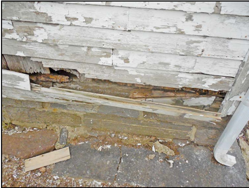
Photo P11 – Close up of southeast corner sill and post water damage.
