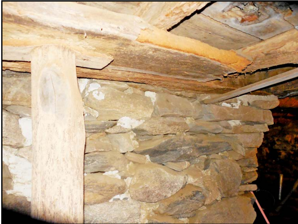
Photo P03 – Timber joists and beams with powder post beetle damage. Note temporary shoring.
