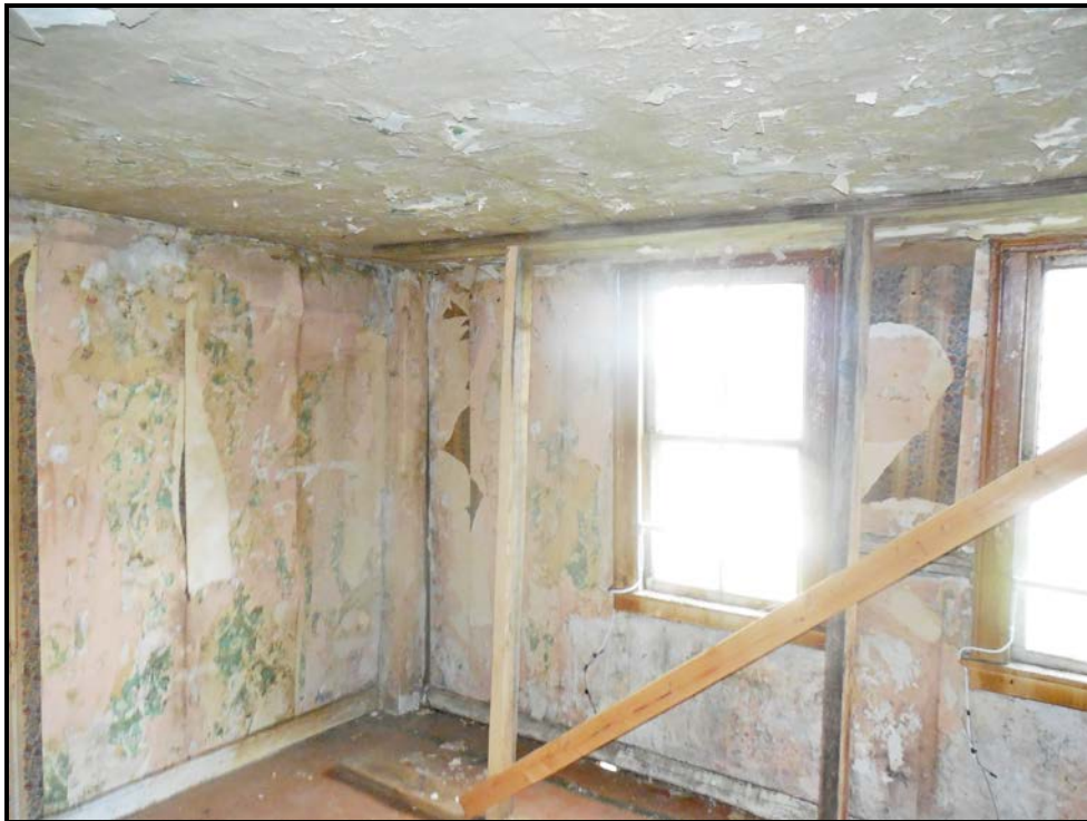
Photo P05 – Front parlor (at south east corner) with sill/wall planking base damage and movements
