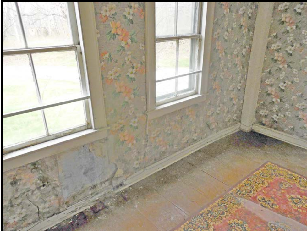
Photo P07 – Moisture/damage at sill line in southwest parlor front wall.
